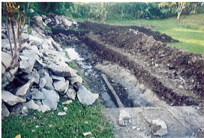
Photo 8.5: Septic tank discharge problem into unsuitable soil conditions
