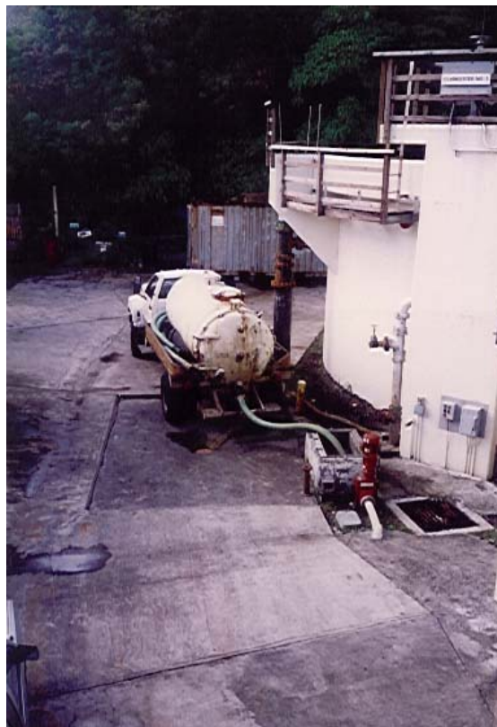
Photo 8.3: Disposal of septic tank solids into Clarigester in American Samoa
